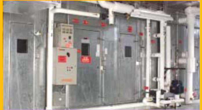
Air handling units
